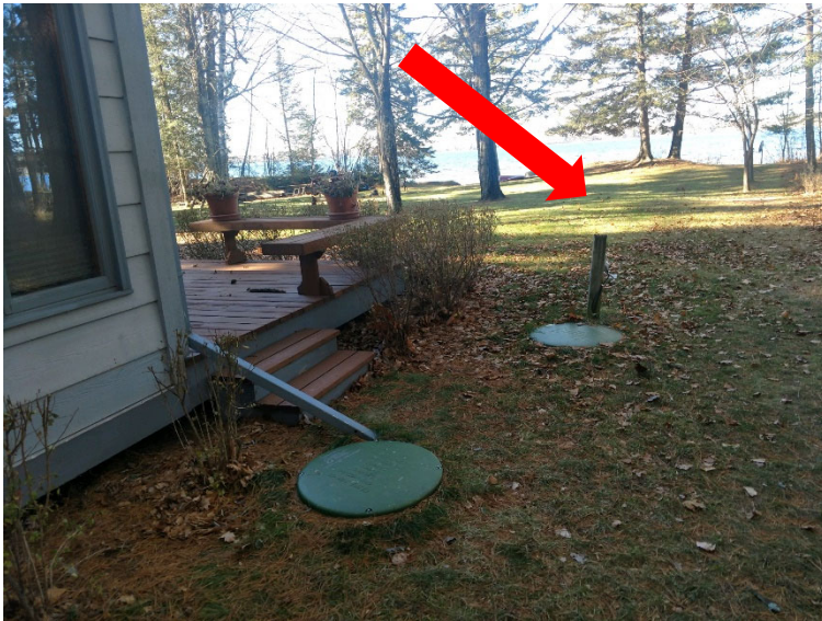
Existing 1250 combo to be reused for septic capacity Arrow points to existing non-compliant drainfield
