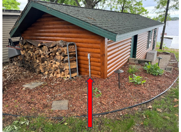
Electrical Connection Location
