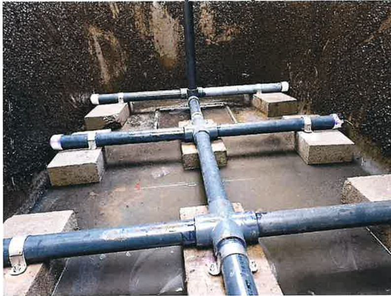
Pic: aeration grid in existing tank
