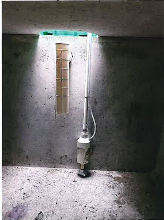
Pic: Air lift sludge return pump and braided hose
