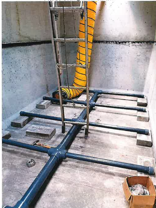
Pic: aeration grid in new tank
