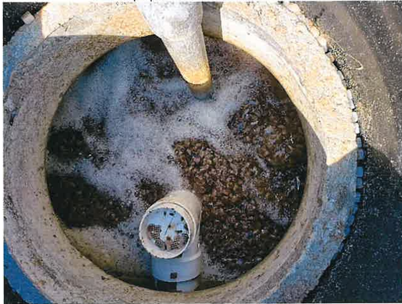
Pic: proper movement in reactor tank
