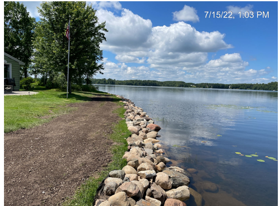
Onsite inspection photo 7/15/22
