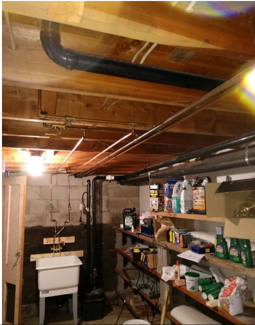
WASHTUB ONLY WHICH IS CONNECTED TO A PUMP THAT GOES INTO THE SEPTIC SYSTEM.
