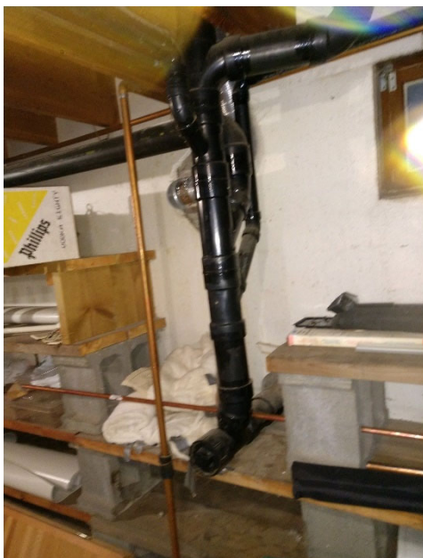
NEWER PLUMBING THAT ALSO GOES OUT TO THE SEPTIC SYSTEM ON ITS OWN 4" LINE.
